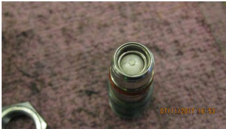
Photo showing dirt build-up on the ball-valve of a disassembled PCCV Sensor.
